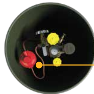
Installed above highest probable water level
